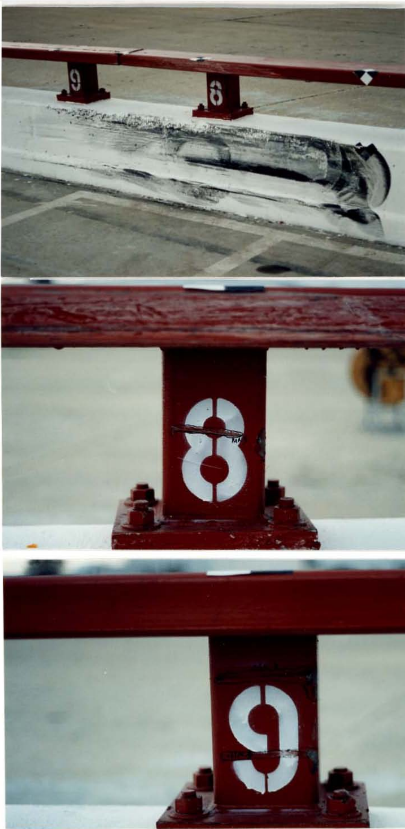
Figure 30. Bridge Rail Damage, Test MN-4.
