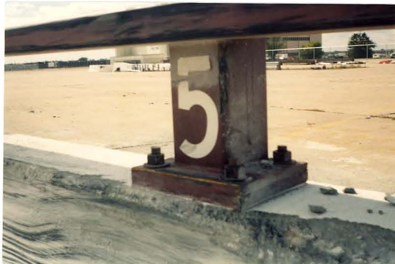
Figure 15. Bridge Rail Damage, Test MN-1.
