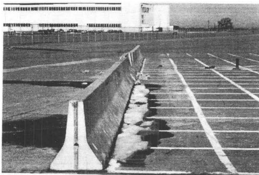
Figure 16. Photographs of the overall damage to the Permanent Precast CMB
