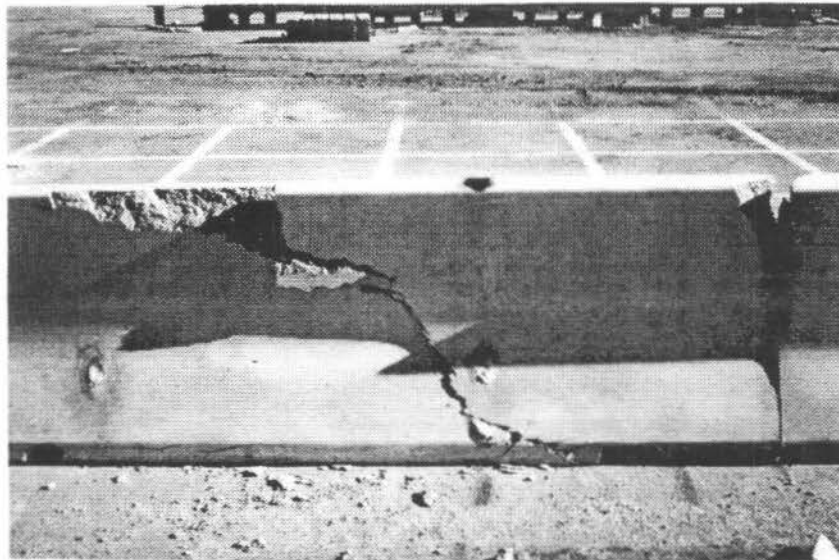
Figure 18. Photographs of the barrier damage at the location of impact (back side)
