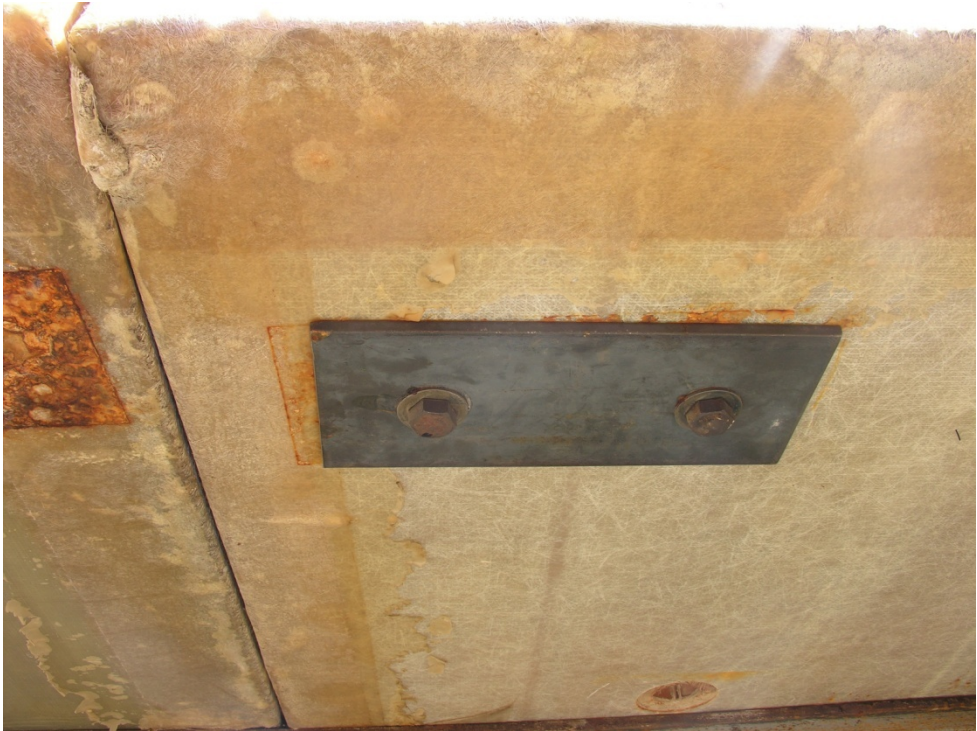
Figure 32. Panel Joints 2 and 3 (Top) and 4 and 5 (Bottom) Damage, Test No. KSFRP-1
