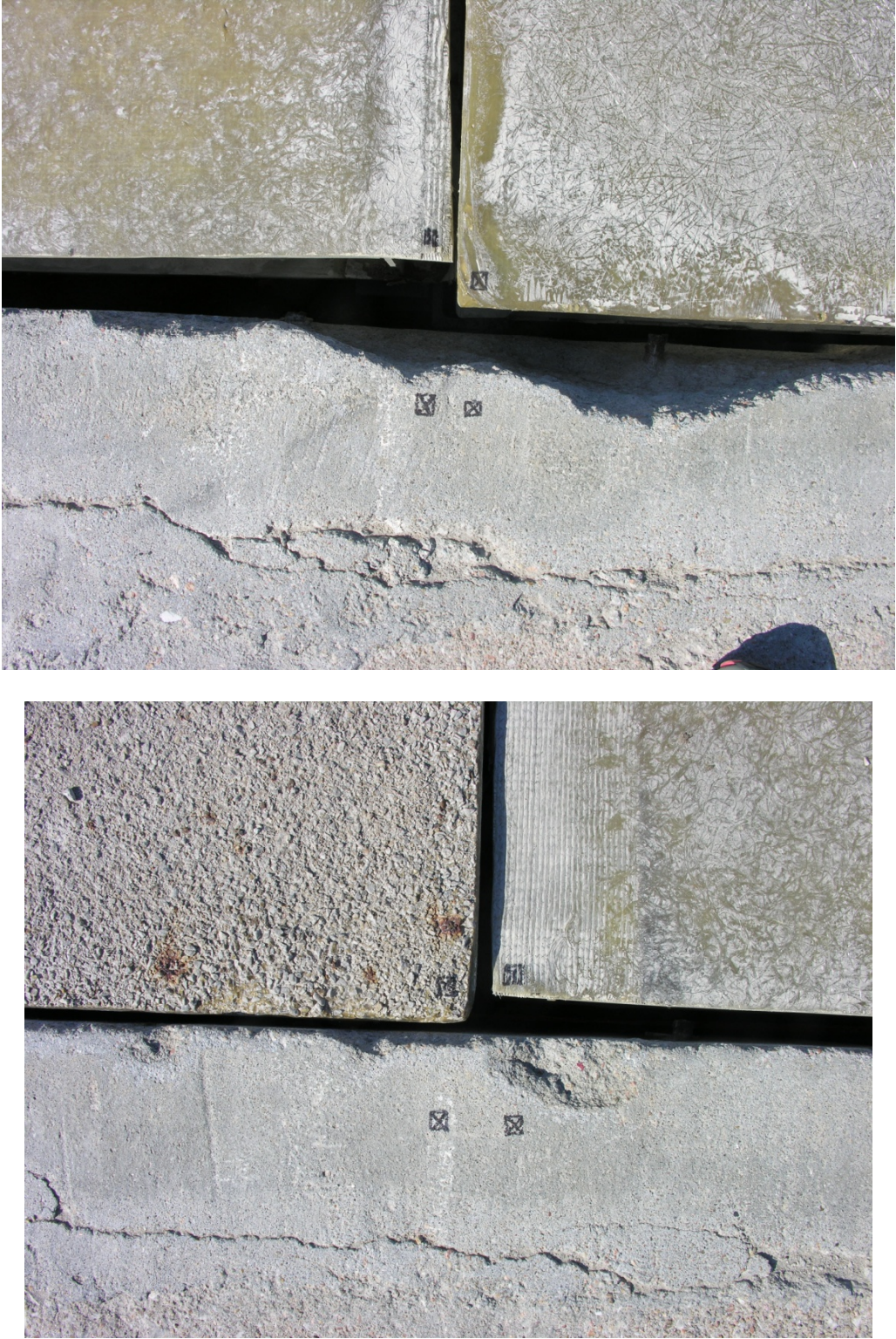
Figure 31. Panel Shift - Joints 3 and 4 (Top) and 4 and 5 (Bottom), Test No. KSFRP-1
