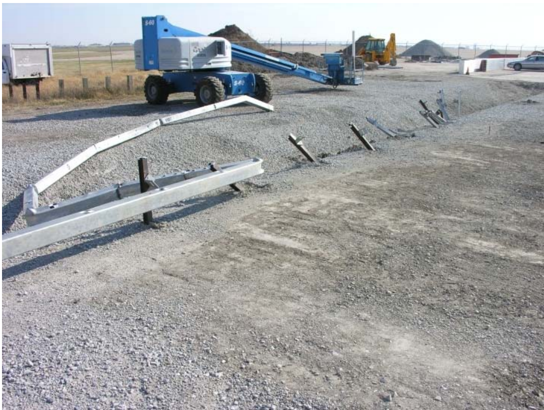
Figure 210. Barrier Damage, Test No. NYBBT-7
