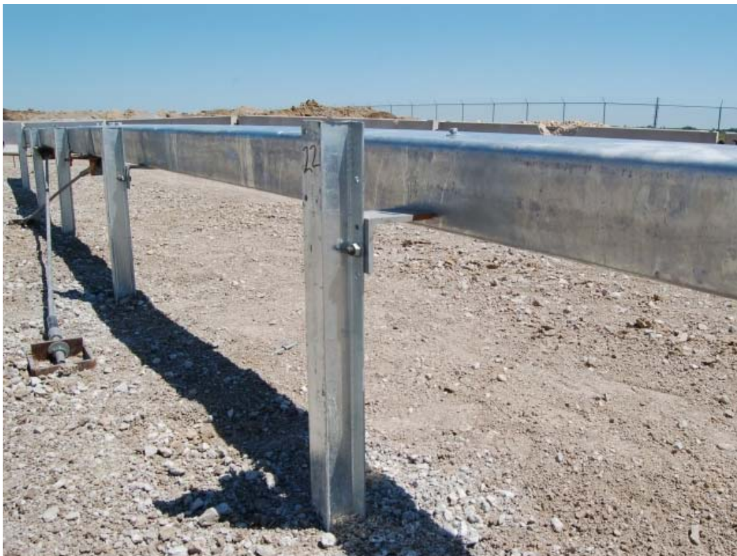
Figure 263. Post Nos. 21 and 22 Damage, Test No. NYBBT-8
