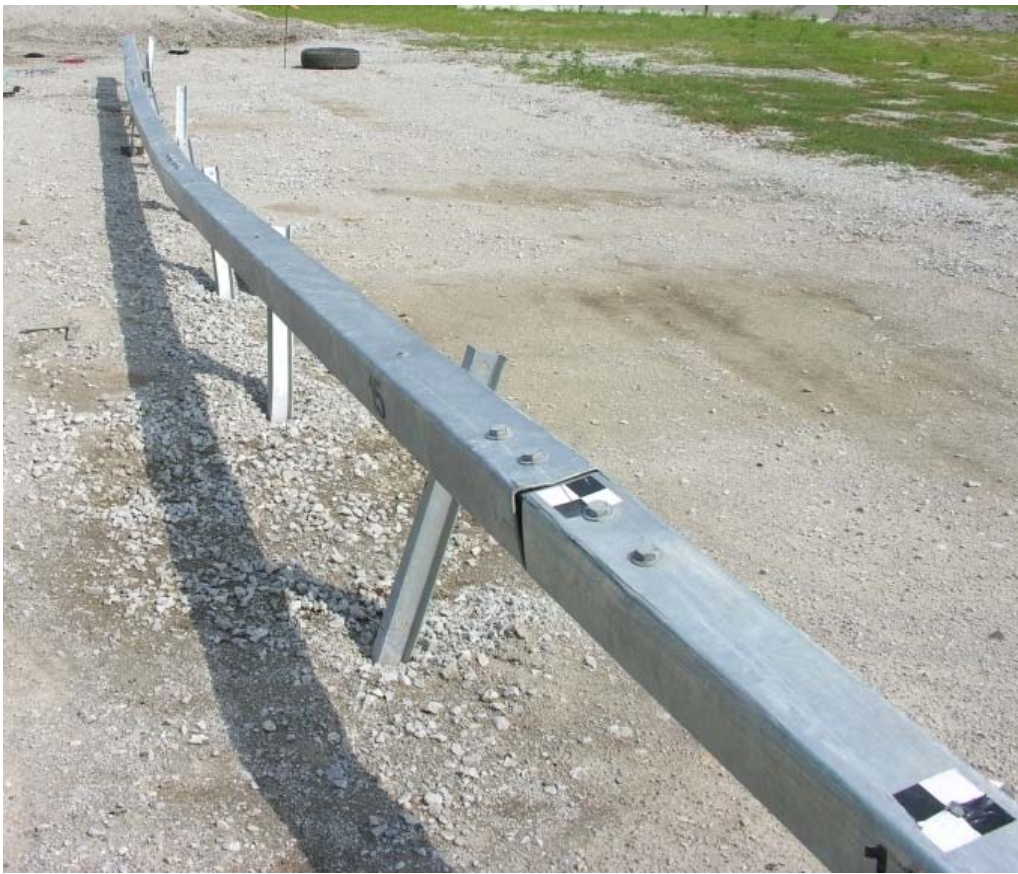
Figure 122. Barrier Damage, Test No. NYBBT-4
