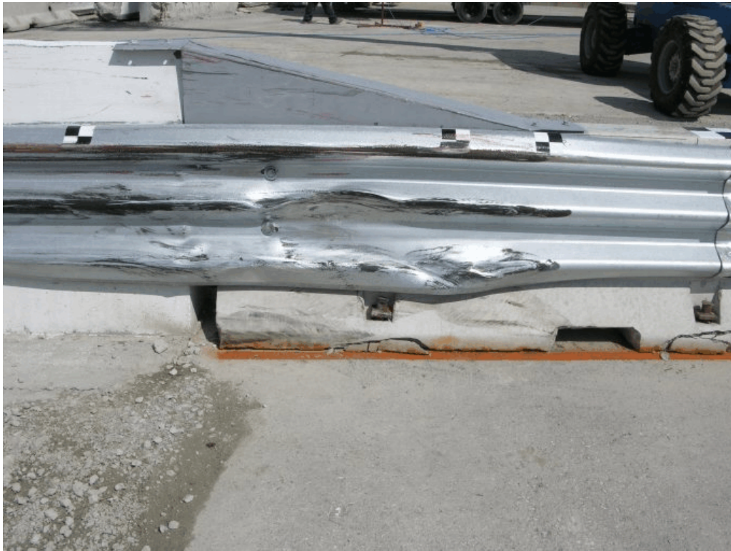
Figure 46. System Damage, Test No. TCBT-1
