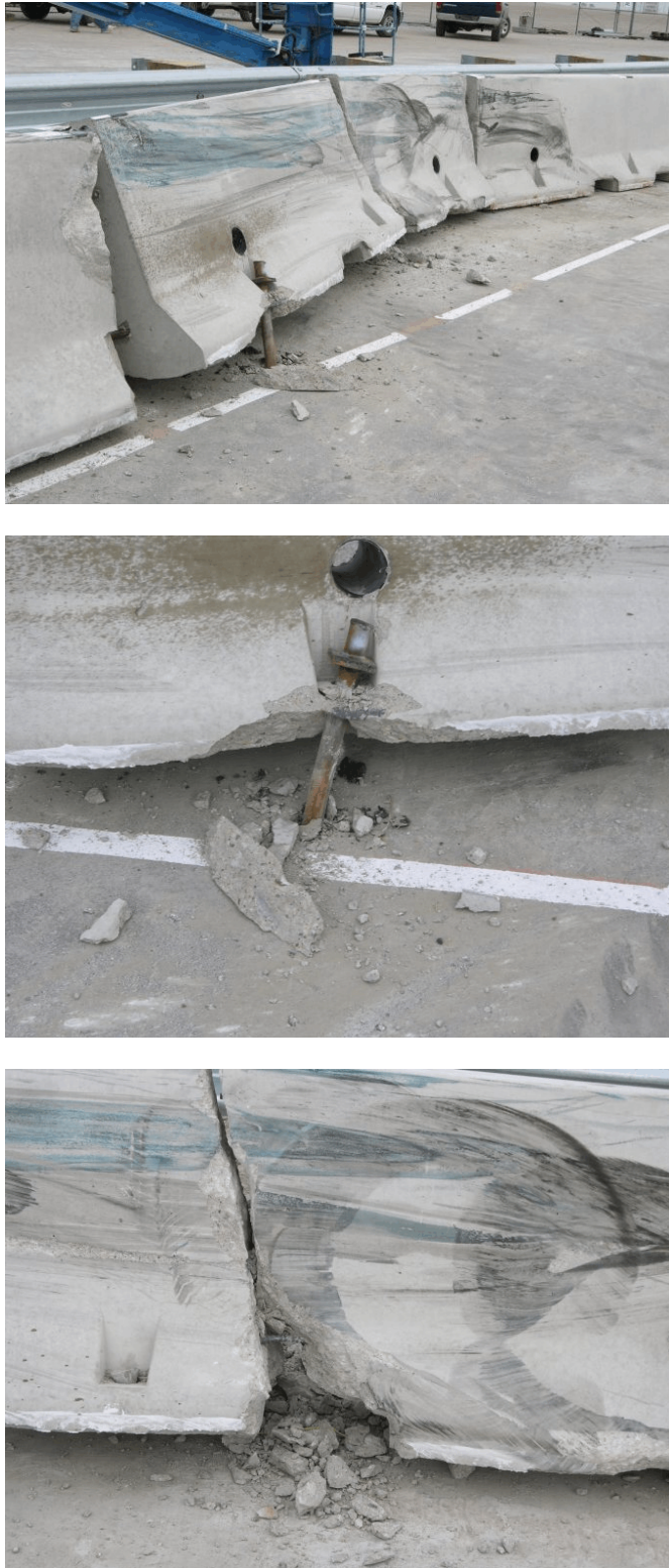
Figure 63. System Damage, Test No. TCBT-2
