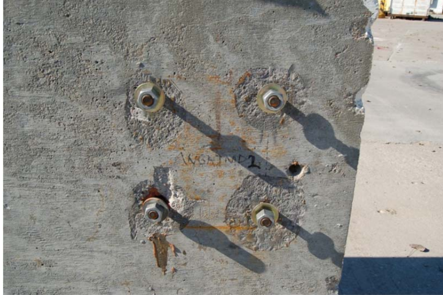
Figure 52. Anchor and Parapet Damage, Test No. WAGTMP-4
