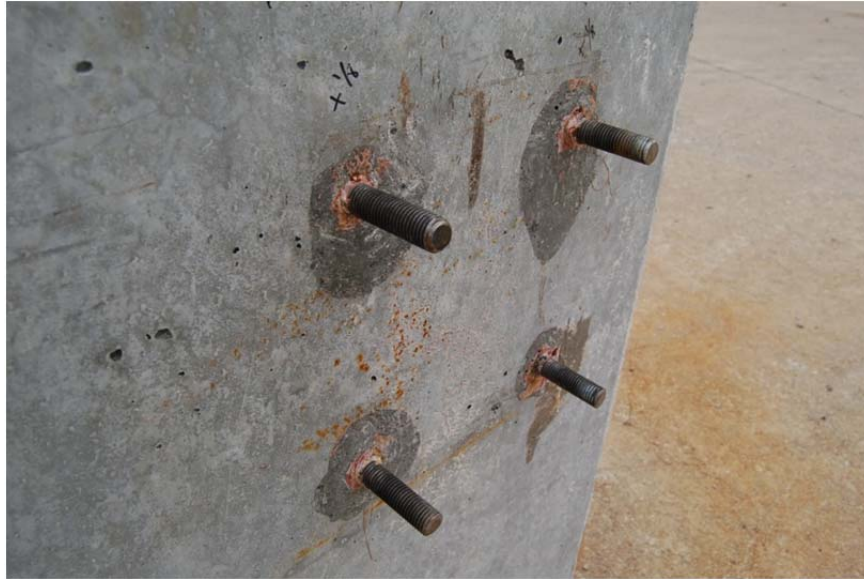
Figure 45. Anchor and Parapet Damage, Test No. WAGTMP-1
