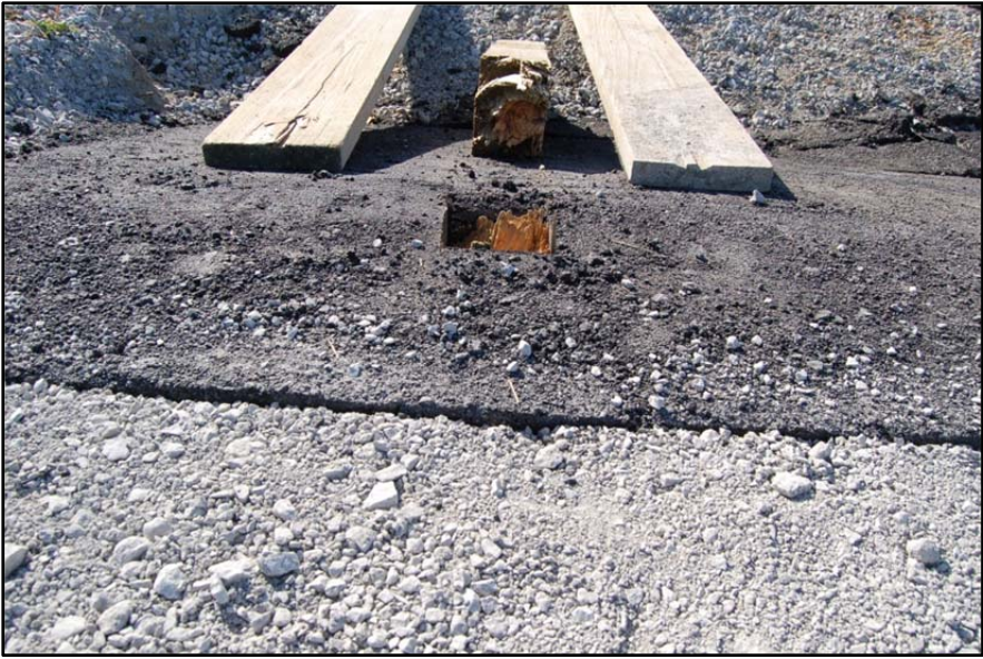
Post After Impact – Front view
