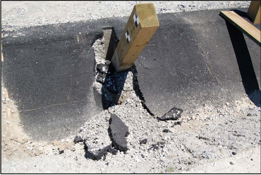
Post After Impact – Asphalt Displacement
