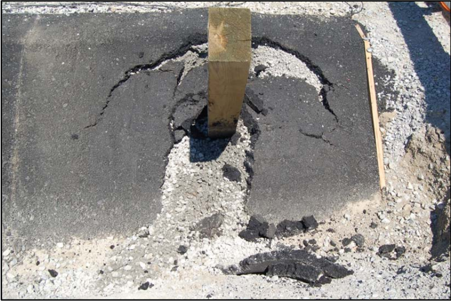
Post After Impact – Asphalt Displacement
