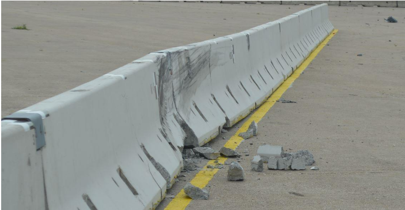
Figure 35. Barrier Nos. 4 and 5 Damage, Test No. NJPCB-7
