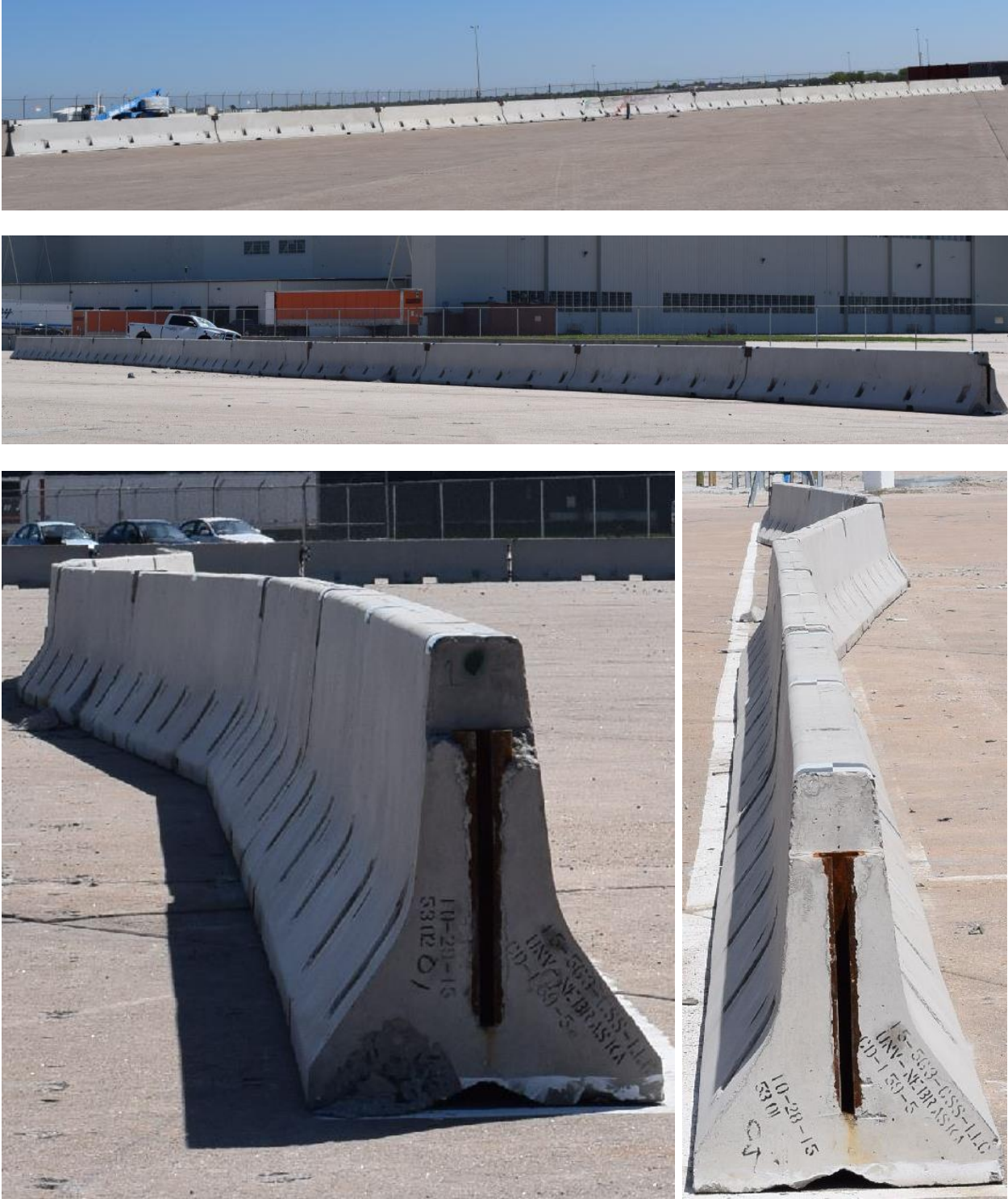
Figure 29. System Damage – Front, Back, Upstream, and Downstream views, Test No. NJPCB-3
