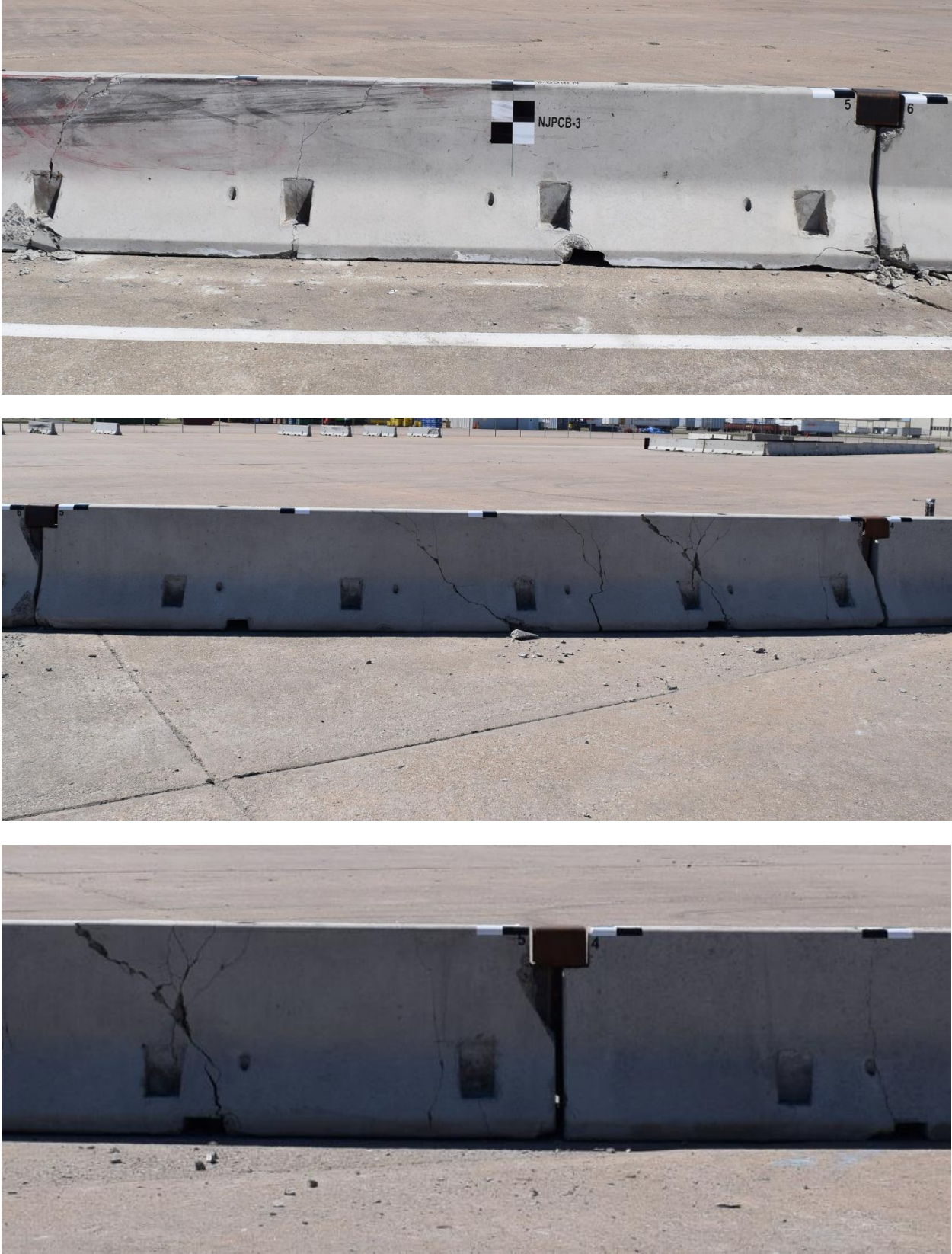
Figure 32. Barrier No. 5 Damage, Test No. NJPCB-3
