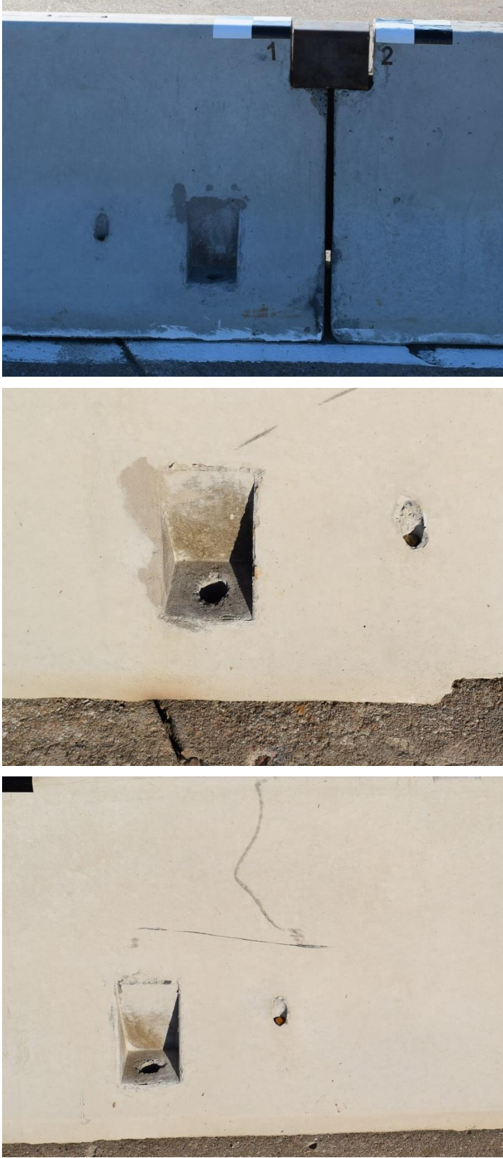
Figure 17. PCB Pin Anchor Recesses (Barrier Nos. 1 and 10), Test No. NJPCB-3
