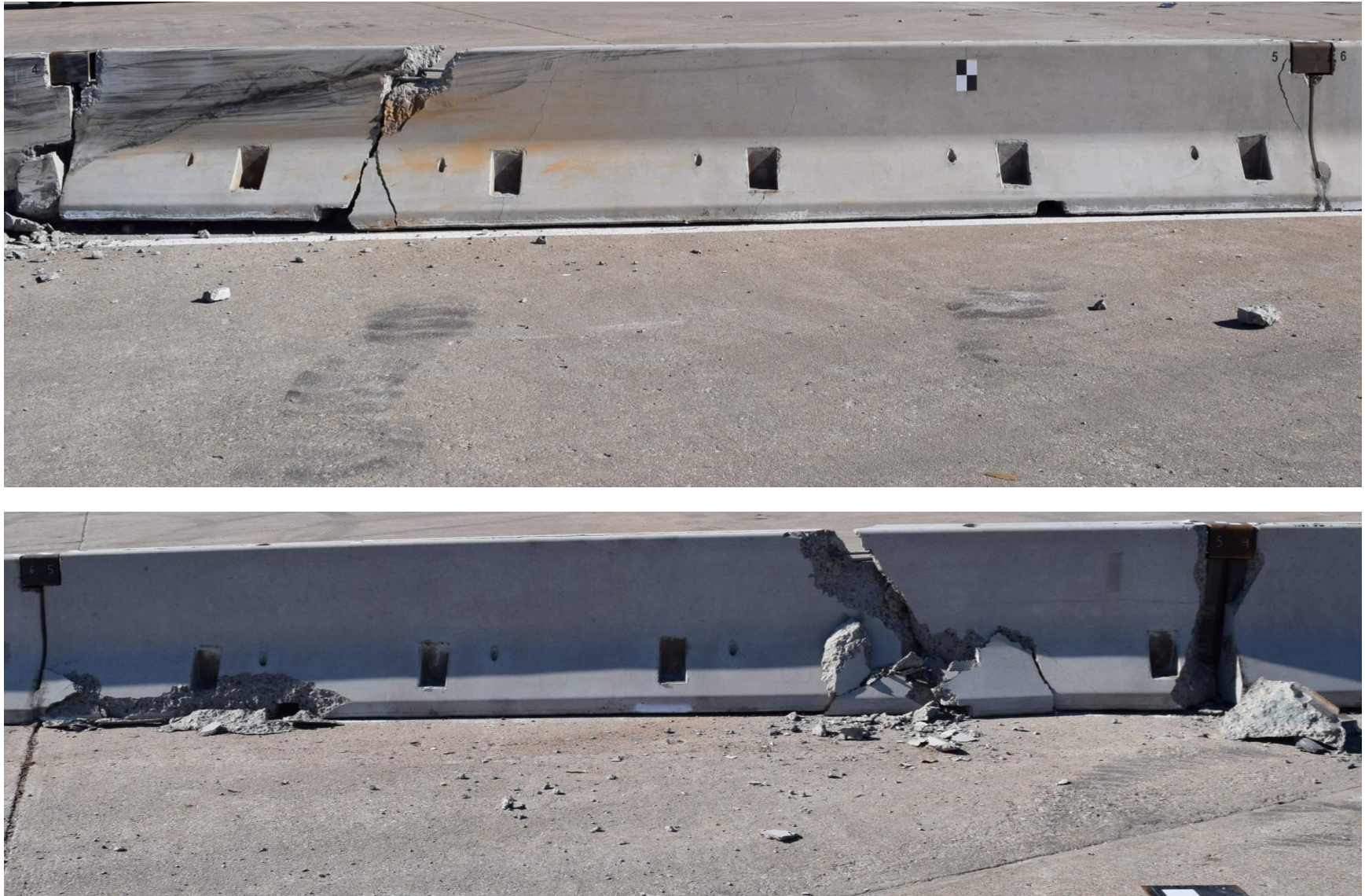
Figure 34. Barrier No. 5 – Traffic and Back Side Damage, Test No. NJPCB-1
