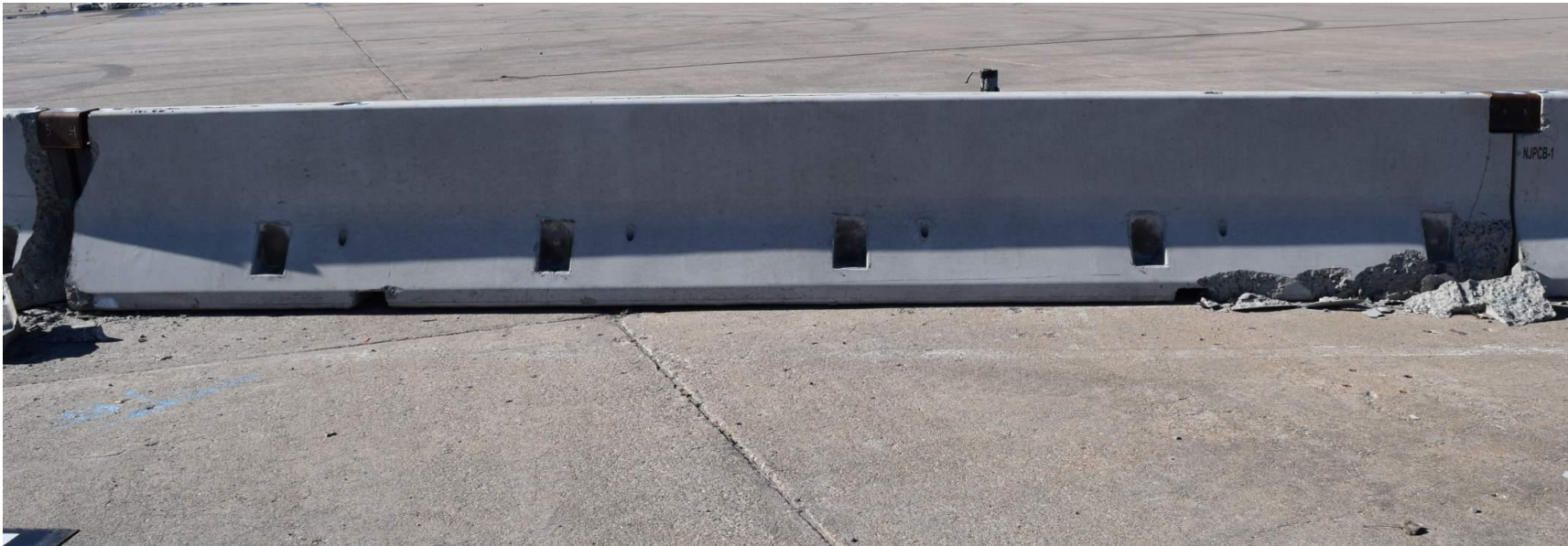
Figure 33. Barrier No. 4 – Traffic and Back Side Damage, Test No. NJPCB-1
