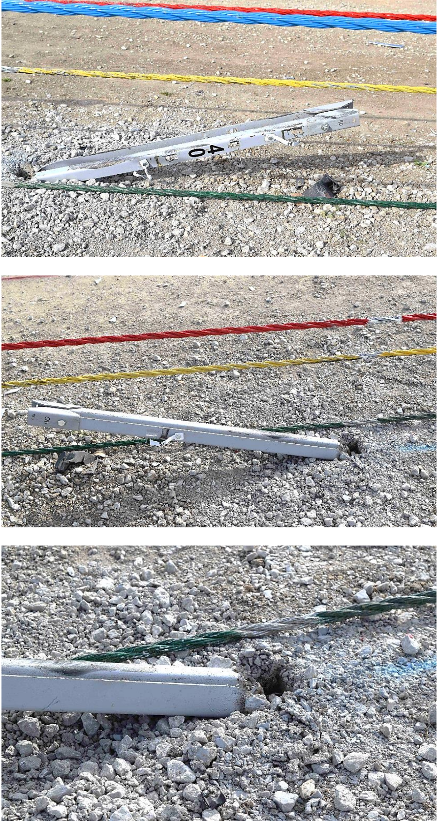
Figure 72. Post No. 40 Damage, Test No. MWP-9
