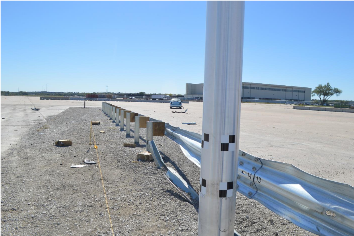
Figure 128. Midwest Guardrail System Damage, Test No. ILT-2
