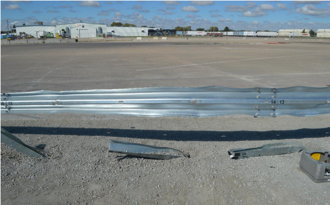
Figure 130. System Damage, Post Nos. 13 through 15, Test No. ILT-2
