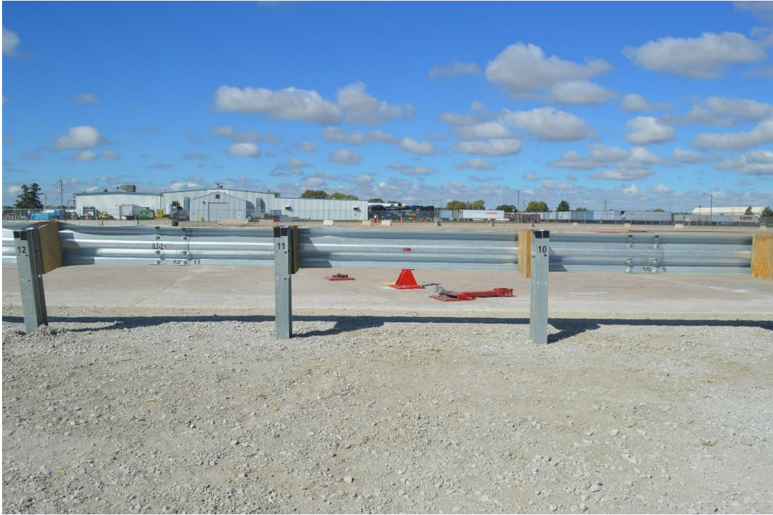
Figure 129. System Damage, Post Nos. 10 through 12, Test No. ILT-2
