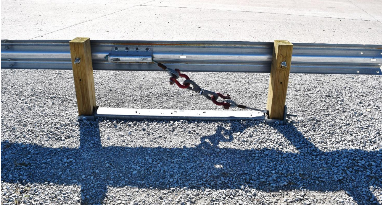
Figure 118. Downstream Anchor Damage, Test No. ILT-1
