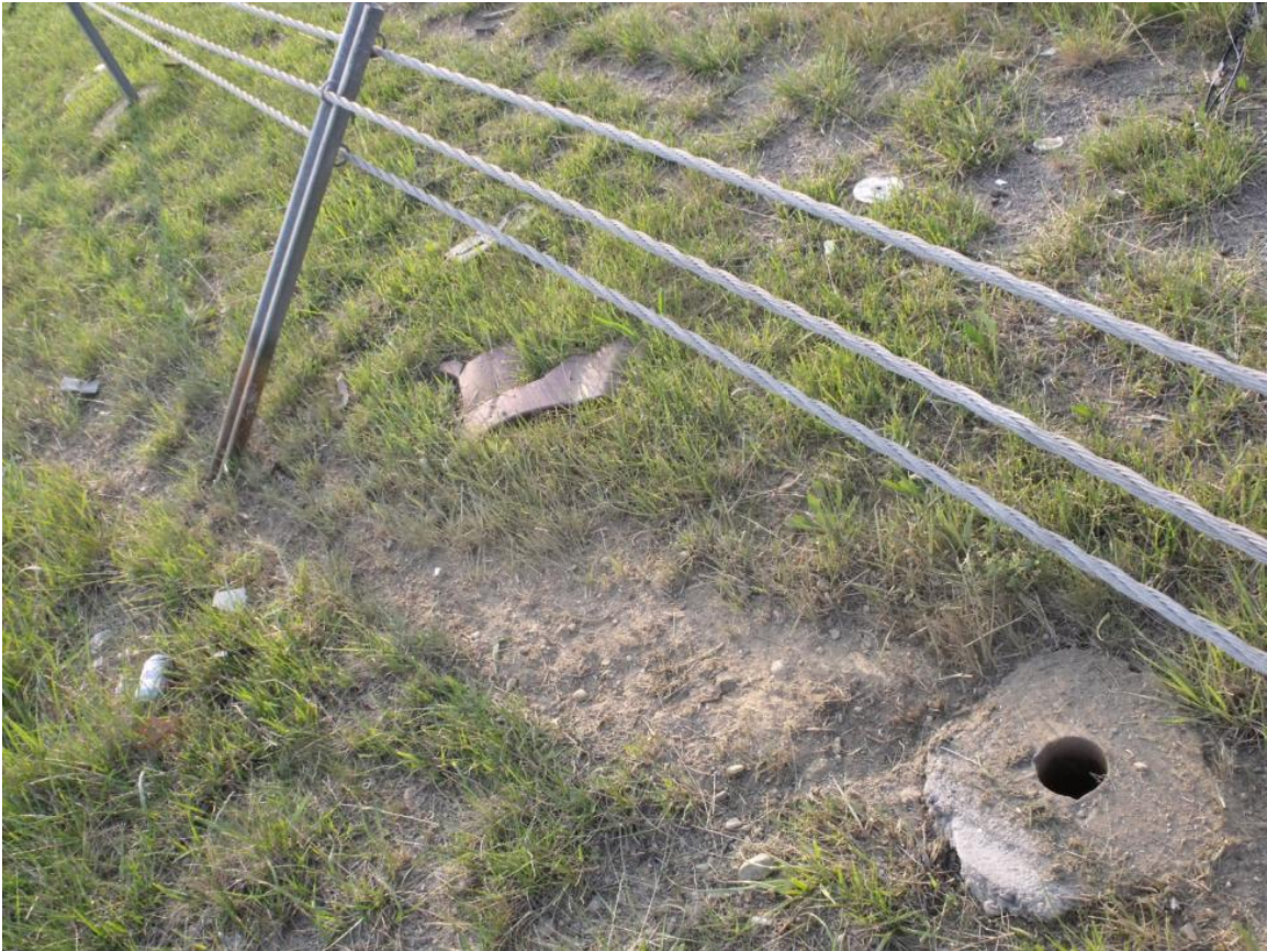
Figure 90. Prying Penetration Crash on Nucor NU-CABLE Barrier
