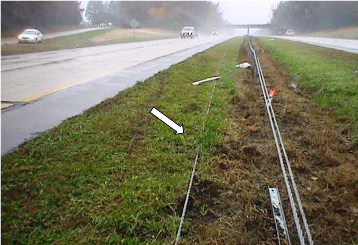
Figure 103. Back Side (Middle) Cable Release from Many Downstream Posts Resulting in Penetration
