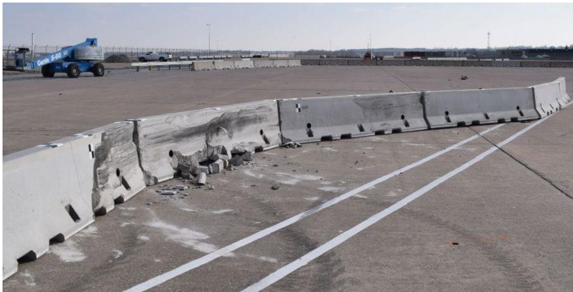
Figure 73. System Deflection and Damage, Test No. NELON-1
