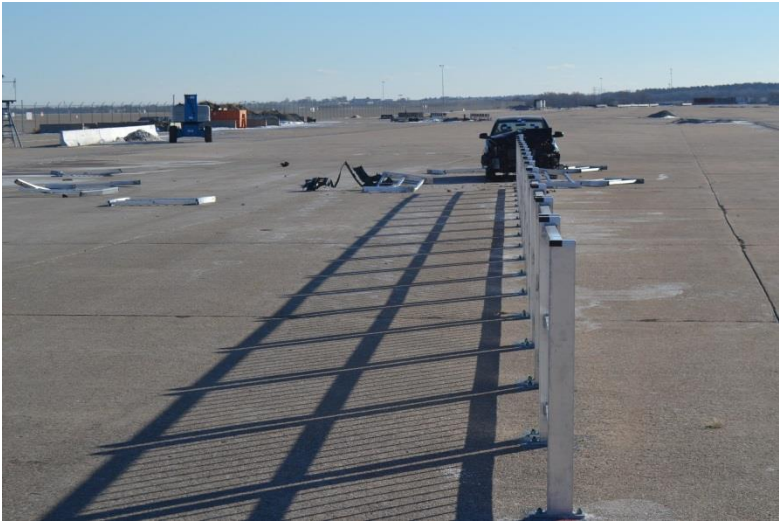
Figure 196. System Damage, Test No. APR-2
