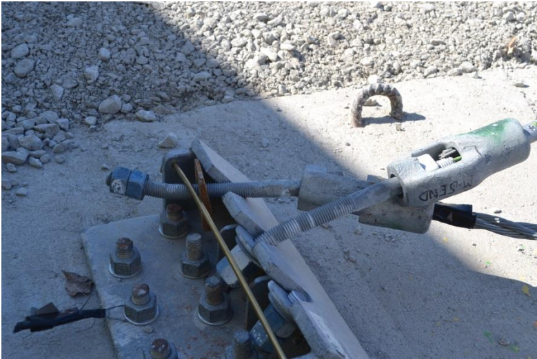
Figure 94. Upstream Anchor Damage, Test No. NYJ-3
