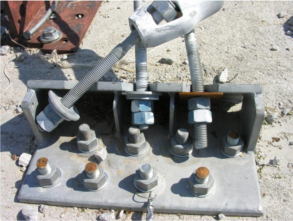
Figure 49. Downstream Anchor Damage, Test No. NYJ-1
