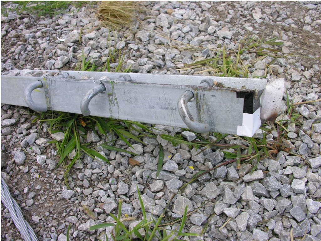
Figure 84. J-Bolt Damage at Post Nos. 18 and 19, Test No. NYJ-2
