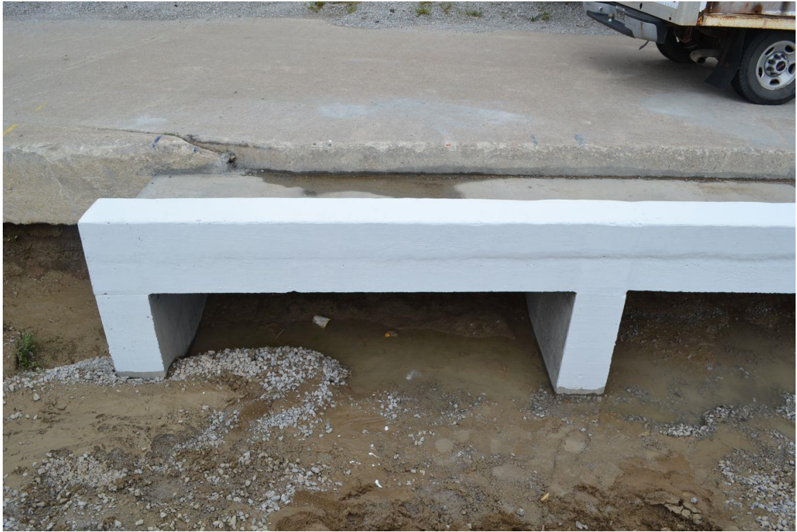
Figure 11. Simulated Culvert Photographs
