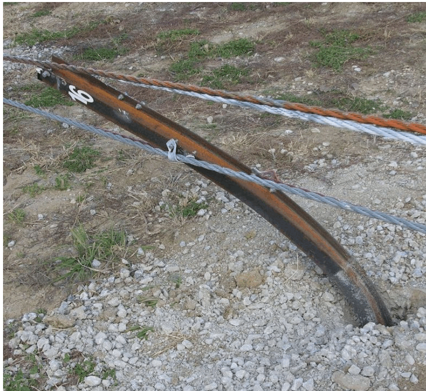
Figure 41. Posts Nos. 14-16 Damage, Test No. 4CMB-1
