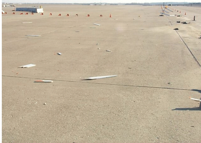
Figure 40. Overall Damage and Final Positions, Test MI-2
