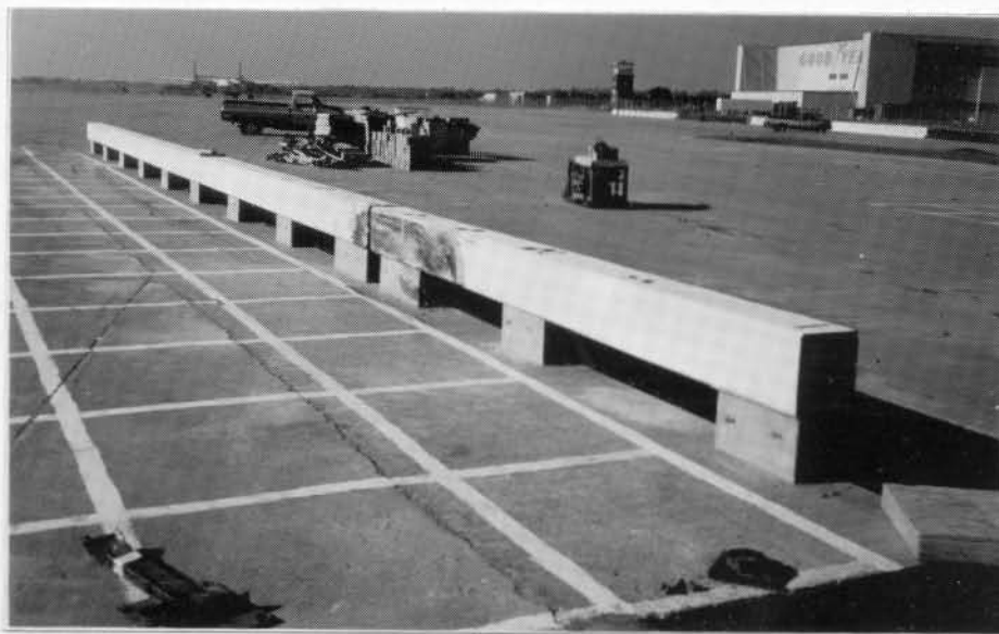
FIGURE 32. Bridge Rail Damage, NEOCR-1
