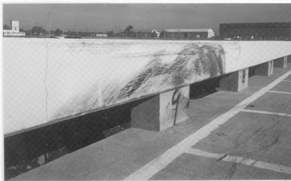
FIGURE 39. Bridge Rail Damage, NEOCR-2
